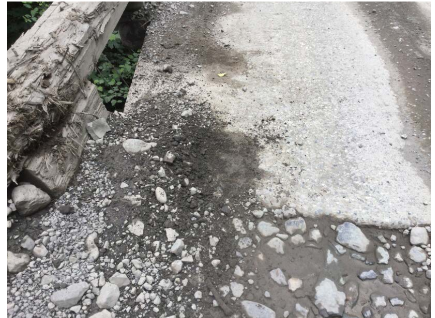
Grout pockets are wearing up to 20 mm in some locations
