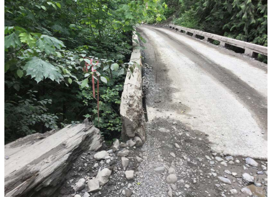
Damage to left downstream guardrail
