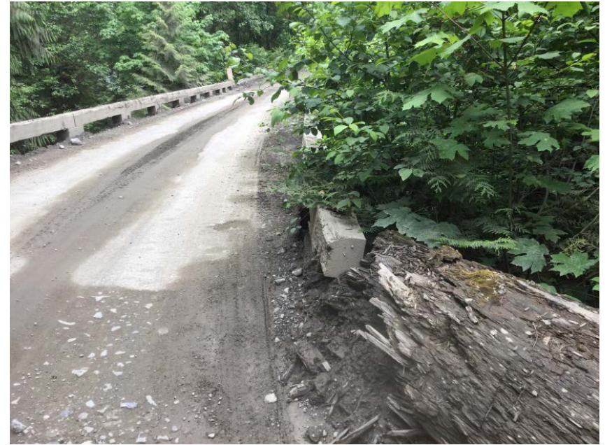
Right downstream guardrail damage
