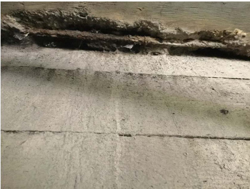
Damage under first panel on right approach
