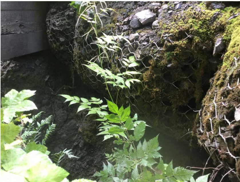
Left downstream gabion wall - up to 500mm erosion under gabions
